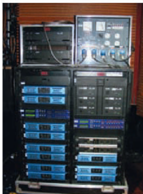
MC2 amplifiers, XTA DP448s and d&b E-Pak units
