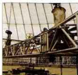
The Tomcat truss, ready for the 'big lift' by Unusual Rigging PHOTOS: MIKE LETHBY
