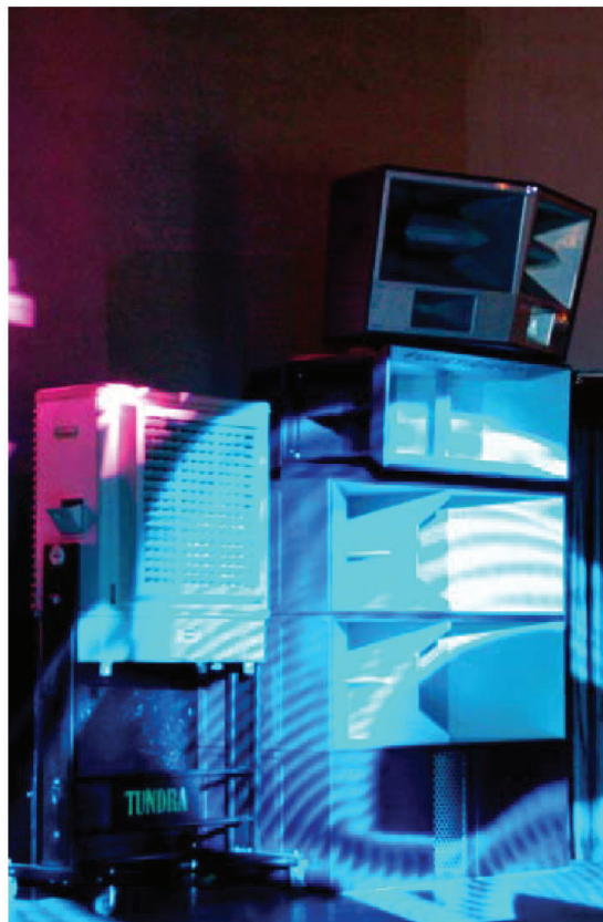
Funktion One Dance Stacks installed in The Club
