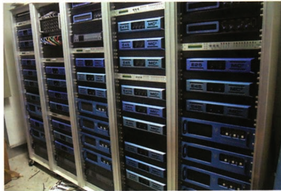
MC 2 amplifiers are crammed into the rack-room
